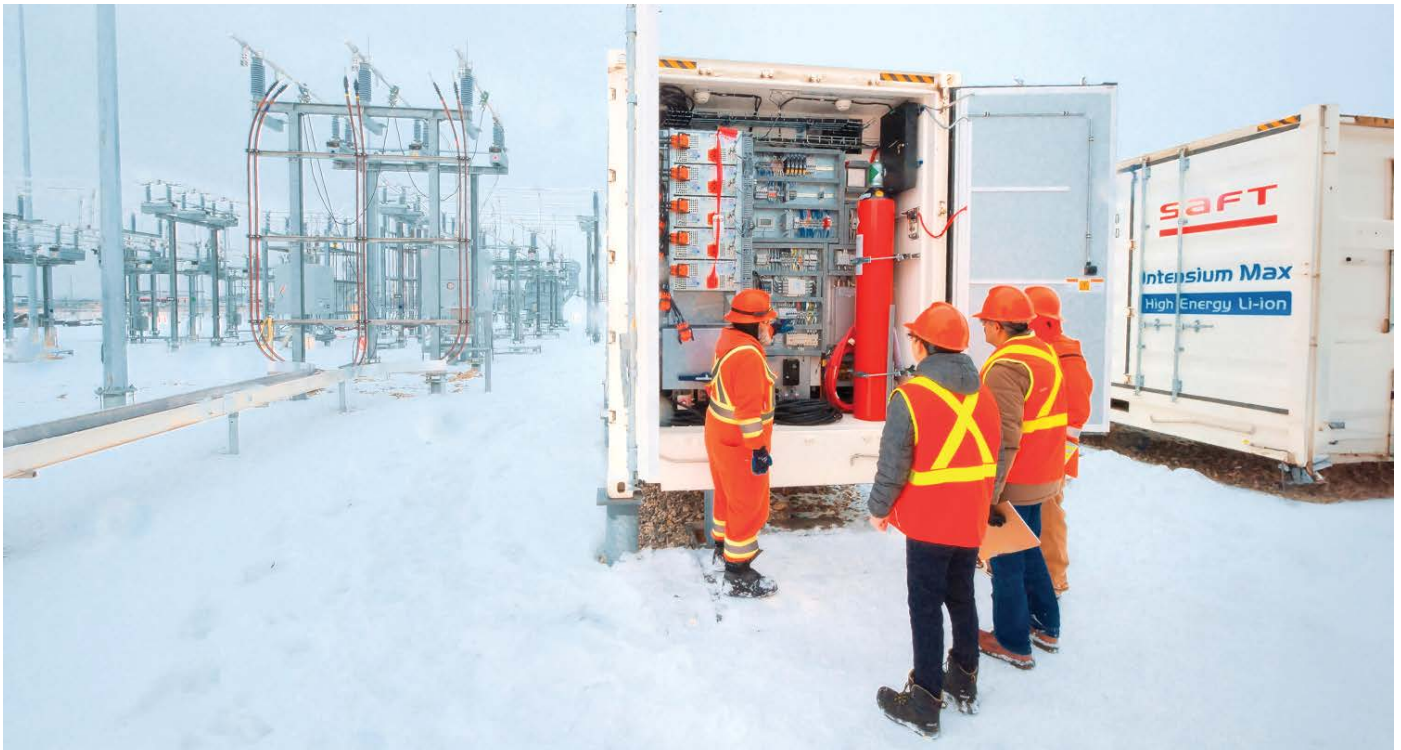
SASKPOWER'S FIRST UTILITY-SCALE BATTERY ENERGY STORAGE SYSTEM IS LOCATED IN REGINA
