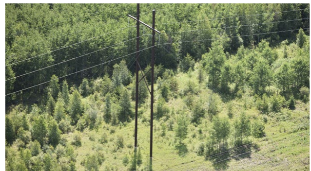
A weathering steel guyed Y structure (top) and a weathering steel H-Frame structure.
